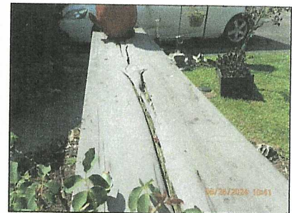
2036 - Entry wall cap deteriorated.
