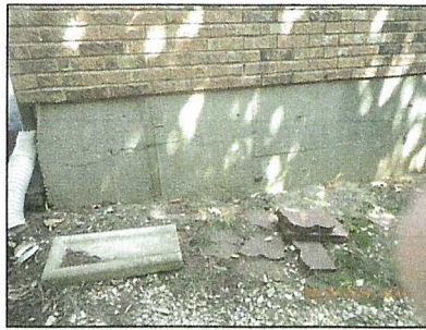
2026 - Cracked foundation wall.
