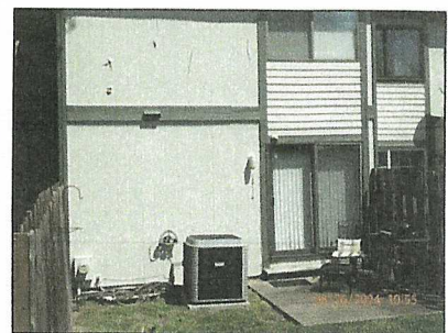
Peeling paint at the rear of the building
