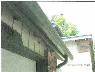
12126 - Bent and damaged gutter.
