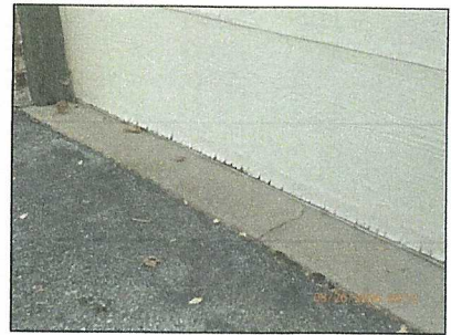
2026 - Garage door deteriorated.
