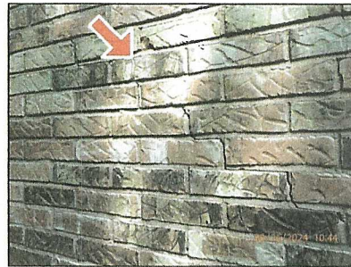
South end of building - stair step cracks in brick work.
