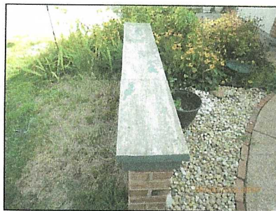
2034 -Entry wall cap deteriorated paint.
