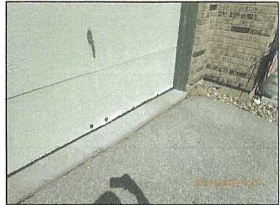
2025 - Garage door deterioration.
