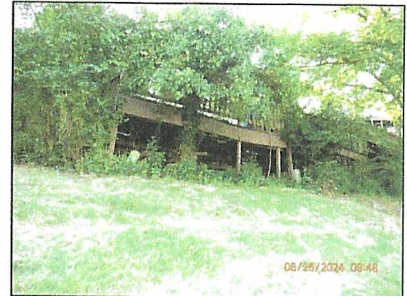
Decks- potential safety issues.
