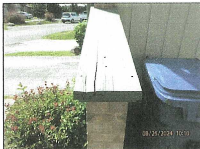
2039 - Deterioration at the wing wall cap.
