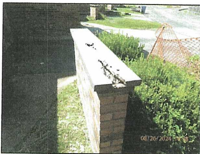
2048 - Entry wall cap deterioration.
