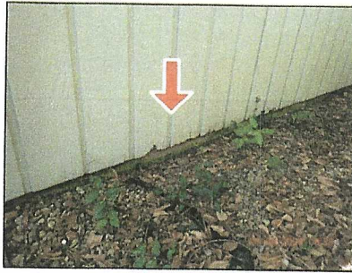
2033- Wood decay at the bottom of the siding.
