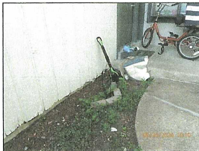
2039 - Bottom edge of siding deterioration.
