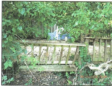
Decks- potential safety issues.
