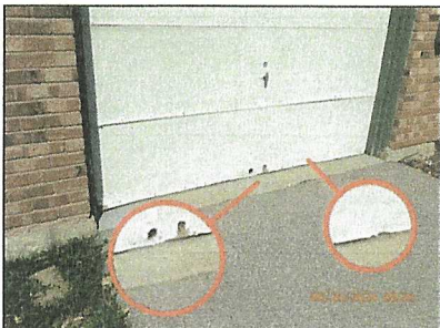
2031 - Deterioration at the garage door.
