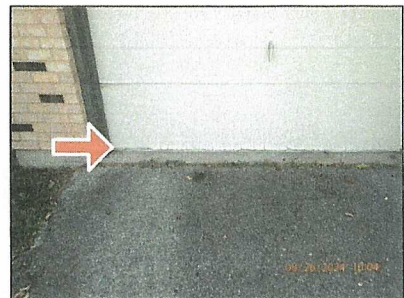
2026 - Deterioration at garage door.
