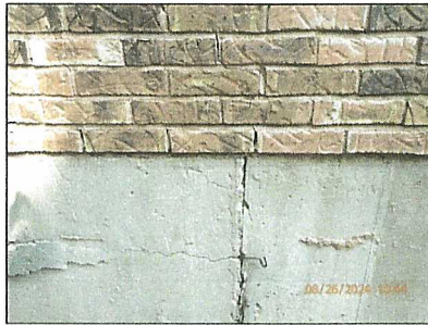
2026 - Cracked foundation wall.
