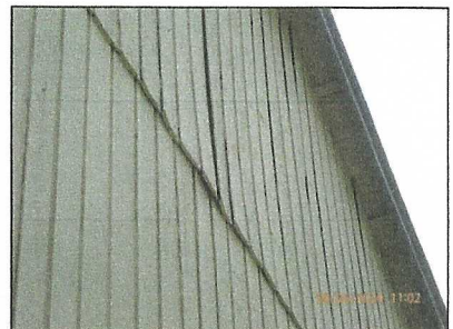
West end of building cupped siding.
