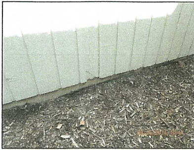
2028 - Minor deterioration at the bottom of the siding.
