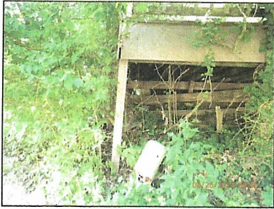
Decks- potential safety issues.
