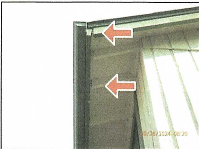
2030 - Loose gutter board.
