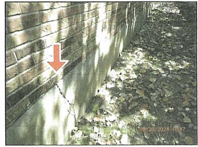
End of building cracked bricks - possible foundation issues.
