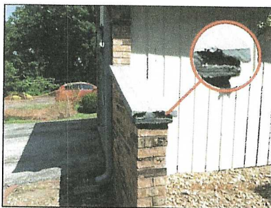
2044 - Wing wall cap wood decay.
