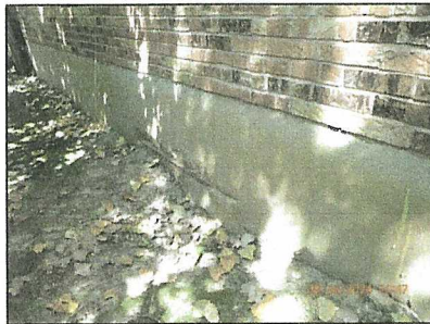
Exposed rebar in foundation wall.
