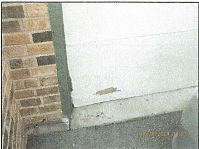
12126 - Deteriorated paint at the garage door.
