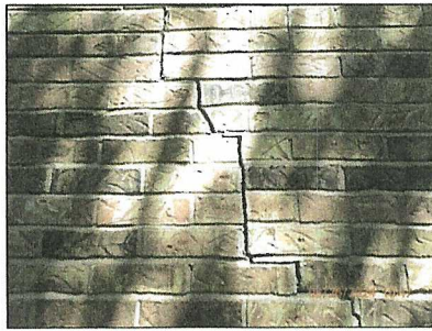
End of building cracked bricks - possible foundation issues.
