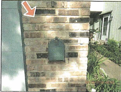
2029 - Sheared and cracked brick.
