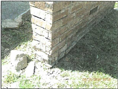
12110 - Entry wall damaged bricks.
