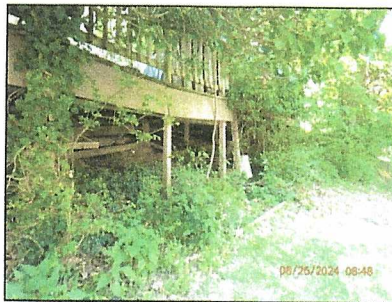
Decks- potential safety issues.
