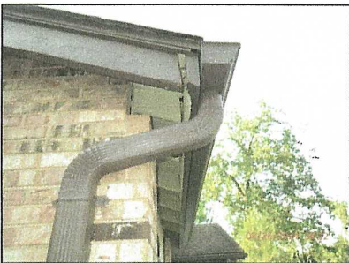
2022 - Loose gutter board.
