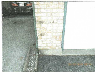
2042 - Sheared bricks at corner.
