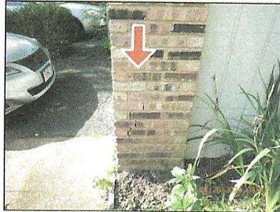
2029 - cracked brick and tuckpointing.
