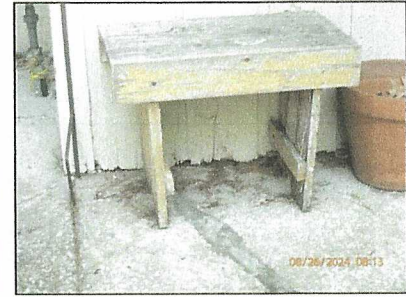
2044 - Deteriorated siding abutting concrete.
