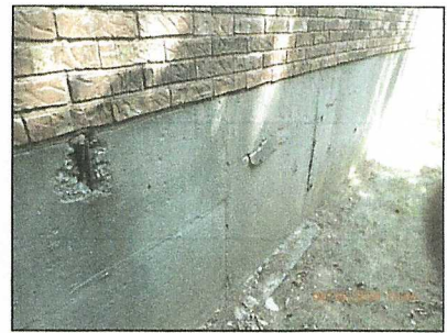
2026 - Exposed rebar in foundation.
