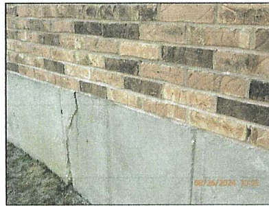
2035 - Cracks in foundation wall.
