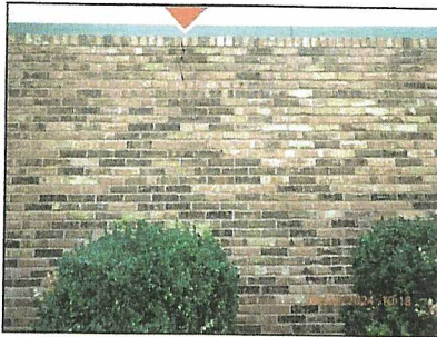
North end of building - sheared bricks
