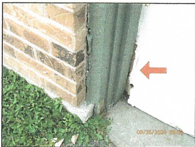
2028 - Deteriorated wood at garage door.
