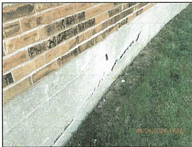
2035 - Cracks in foundation wall.
