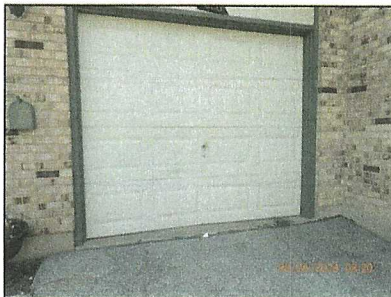
2028 Bent and damaged garage door.
