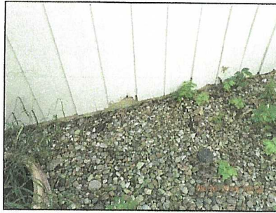
2043 - Deterioration at the bottom of the siding.
