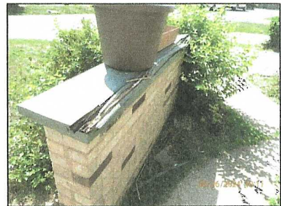
2041 - Entry wall cap deterioration.
