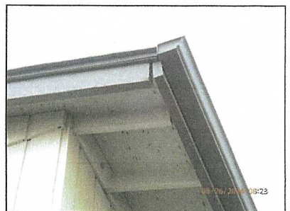
2020 - Loose gutter board.
