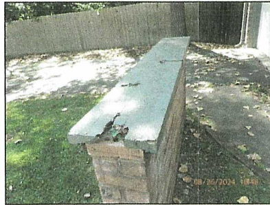
2027 - Deteriorated wood cap.
