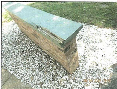
2027 - Damaged cap at entry wall.
