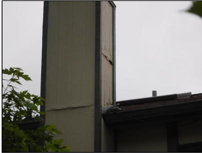
2038 rear - Chimney chase damage.
