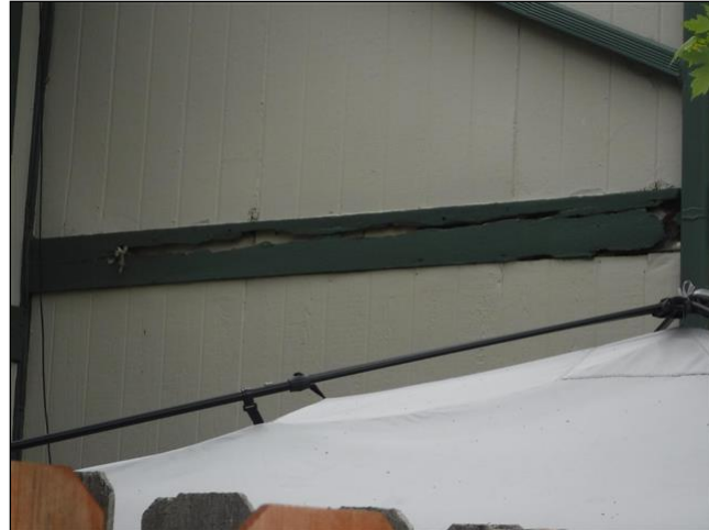
2038 rear - siding trim damage
