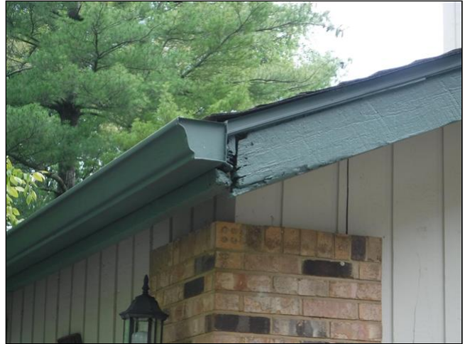
2038 - Rake fascia damage.
