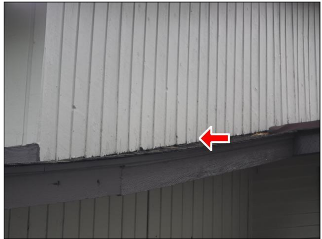
2022 - Minor decay to siding.
