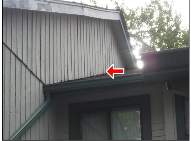
2030 - Minor siding damage.
