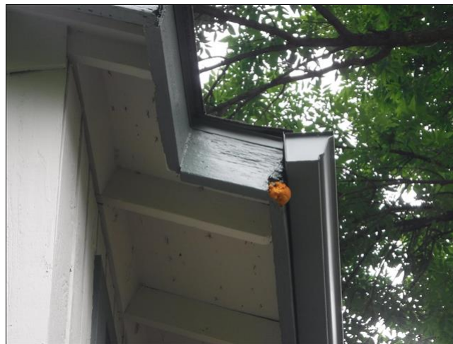
2025 - Damaged rake fascia.
