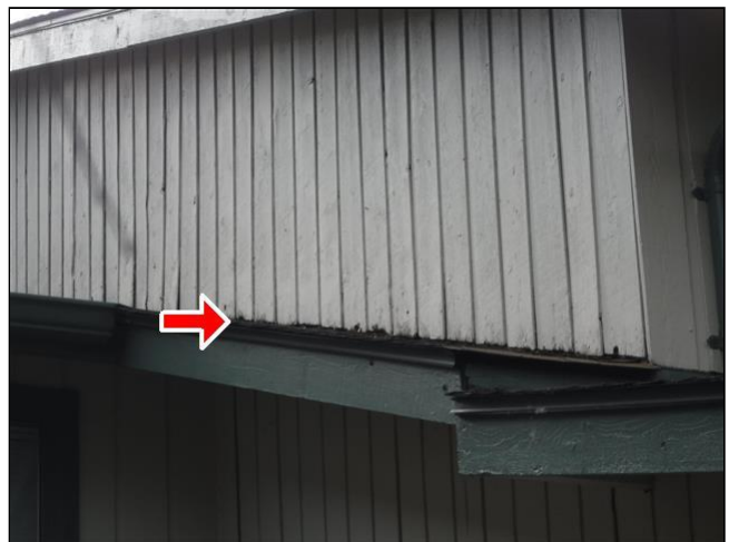
2028 - Minor siding damage.
