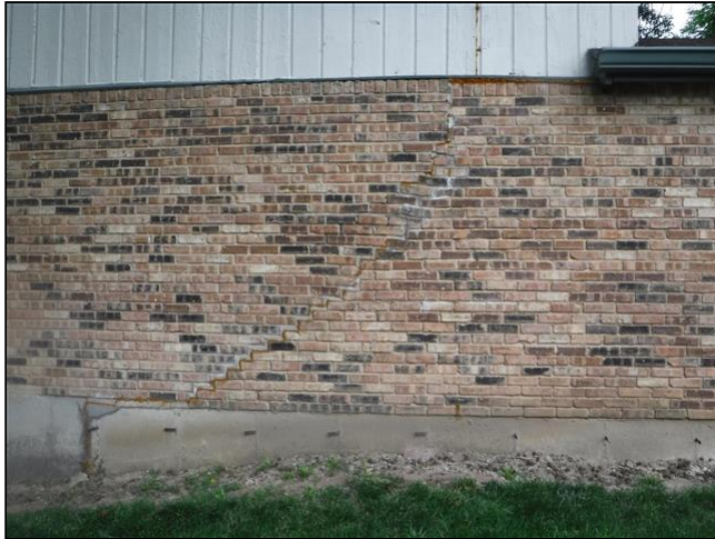
Settlement of building on south side.
