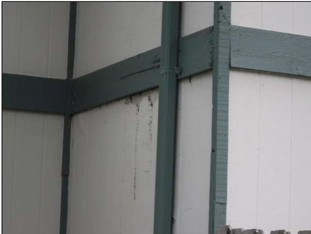
2038 rear - Siding damage.
