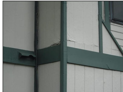
2038 rear - Chimney chase damage.
